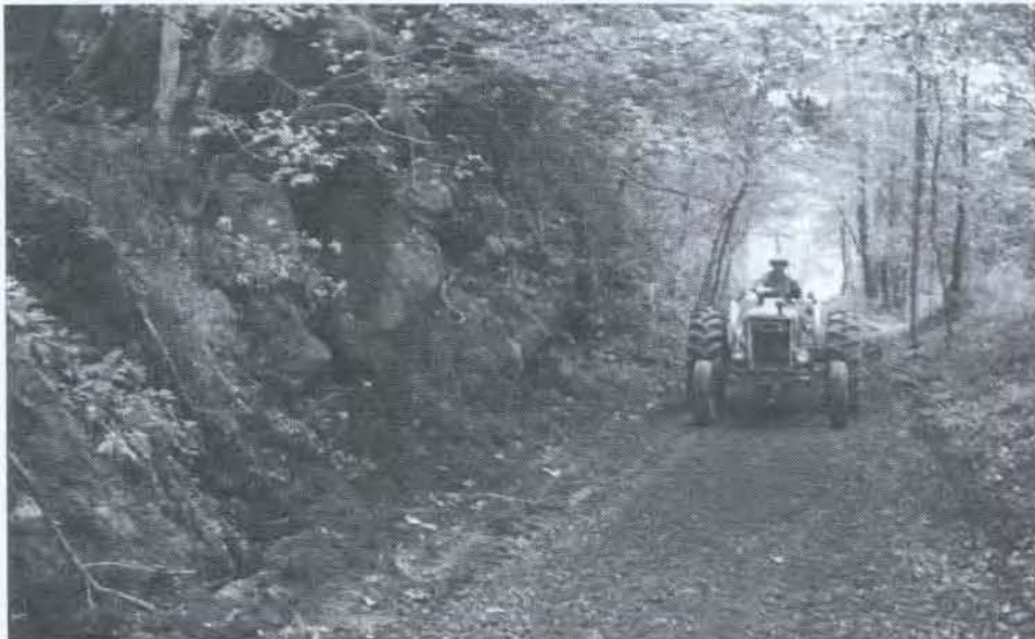
Contractor Jerry Carpenter smooths crushed gravel surface of Lansing's new rail-trail on the former Virginia-Carolina rail bed in Ashe County. A town park is next.
