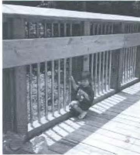
A young hiker checks out the safety features of the Reedy Branch Creek bridge, one of three bridges rebuilt on the Wake County Phase I American Tobacco Trail development.
